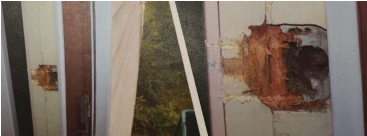
Damage Caused to Door from Crowbar Used During Burglary
